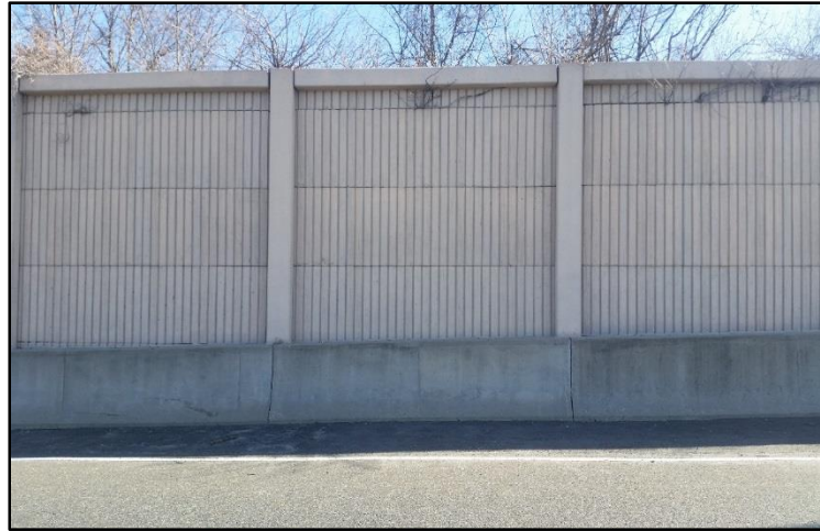
Proposed Noise Walls for I-95 Southbound
